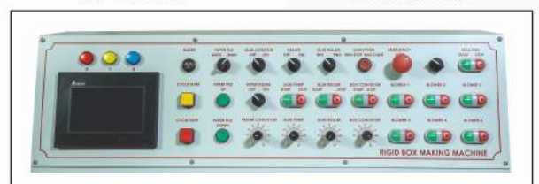
PLC TOUCH CONTROL PANEL
